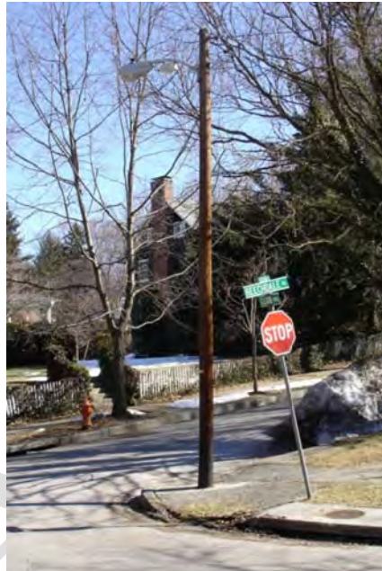
Wooden Pole with Cobra Head Fixture
