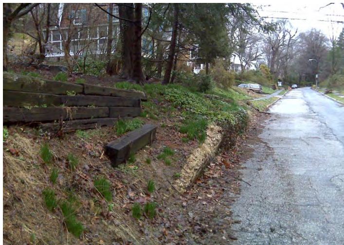
A failing retaining wall within the right-of-way.
