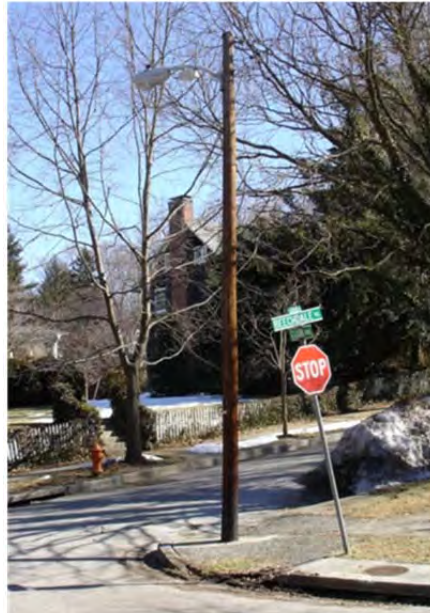
Wooden Pole with Cobra Head Fixture
