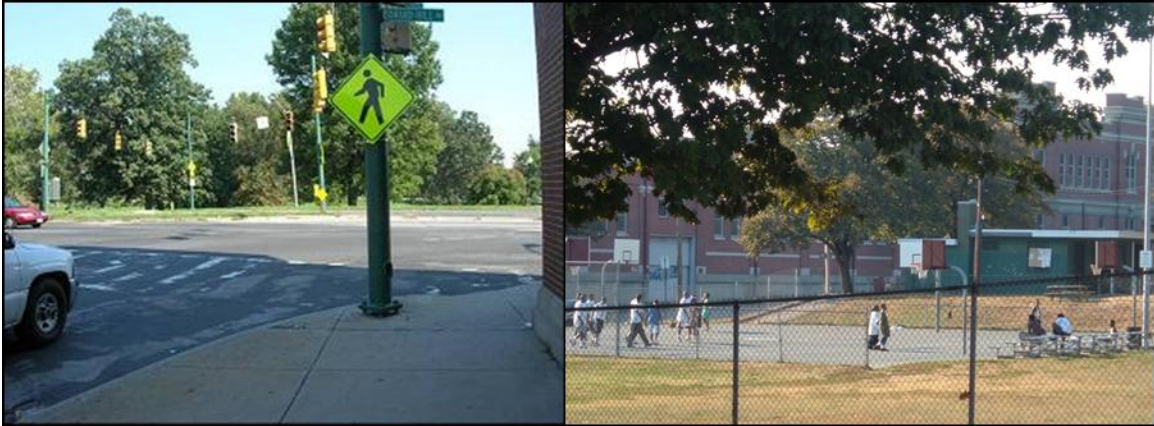
Figure 5: On the left: Worn-out pavement markings at the intersection of Fulton Avenue and Druid Park Lake Drive. On the right: The frequently used Cloverdale Courts.
