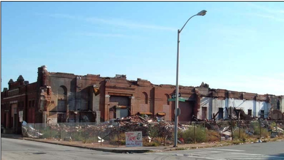
Figure 12: What remains of the former Baltimore Transit Company building after a major fire in 2005.
